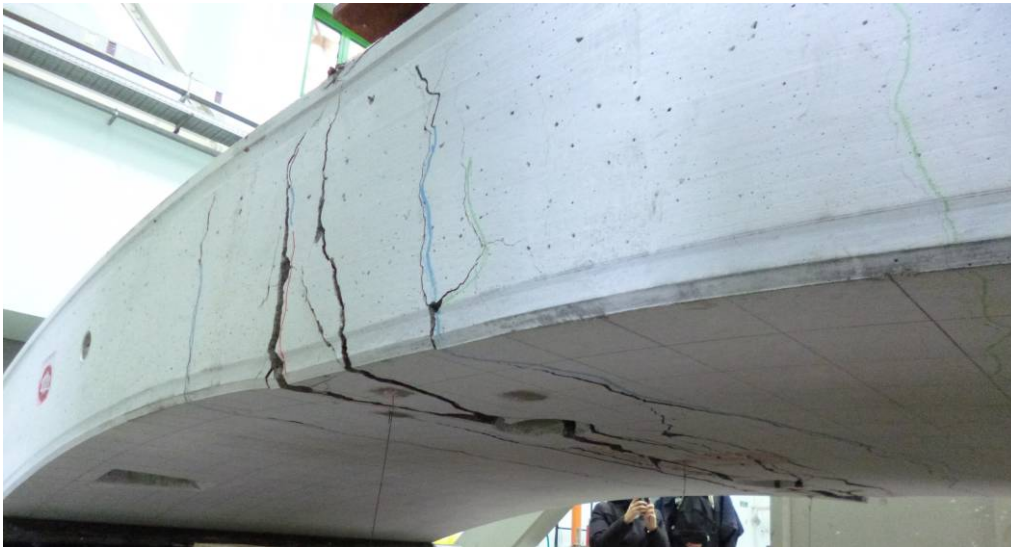
Figure 21. Segment D4: failure stage: intrados surface.
