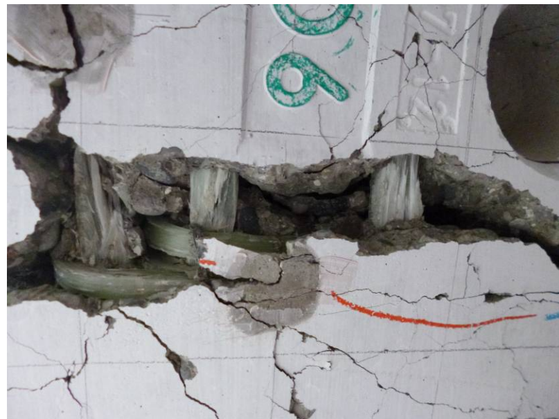
Figure 50. Segment D6: failure stage: intrados surface.
