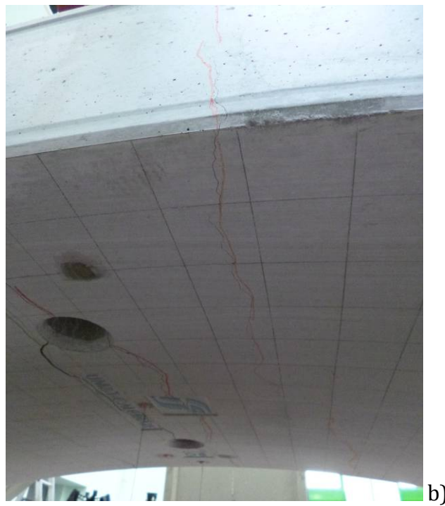
Figure 32. Segment D5: load level of 195 kN – intrados surface
