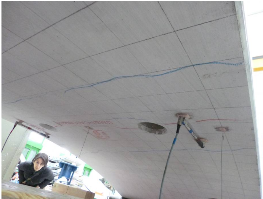
Figure 15. Segment D4: load level of 200 kN, intrados surface
