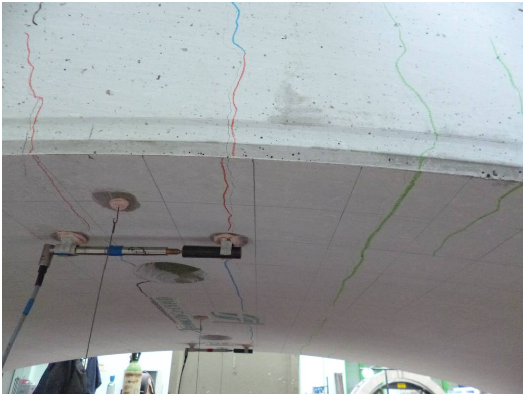
Figure 46. Segment D6: load level of 185 kN – intrados surface
