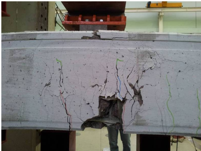
Figure 49. Segment D6: failure stage: left lateral surface.
