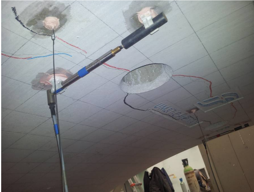
Figure 29. Segment D5: load level of 160 kN, intrados surface
