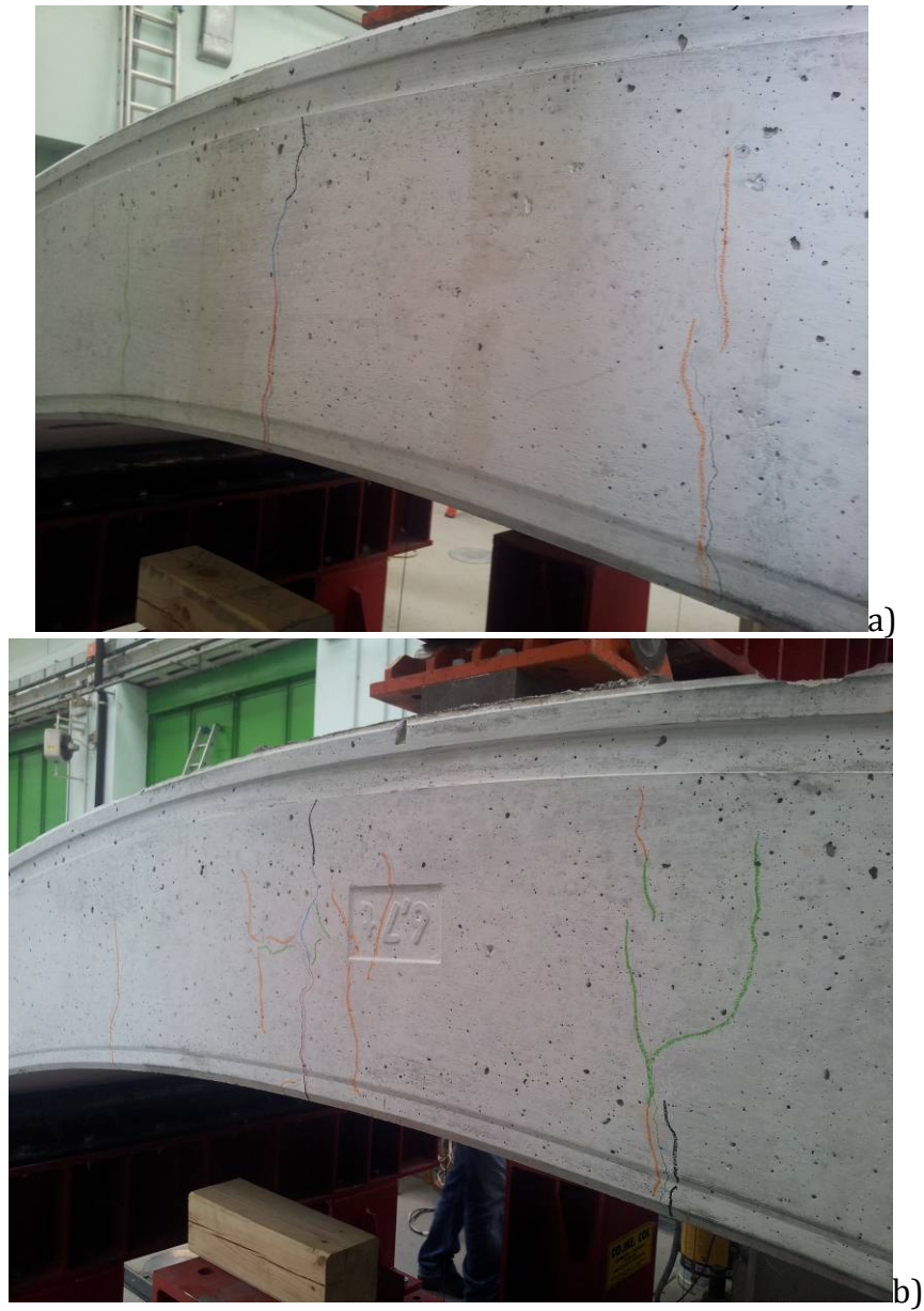
Figure 31. Segment D5: load level of 195 kN; a) left lateral surface, b) right lateral surface.
