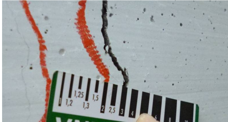
Figure 19. Segment D4: load level of 300 kN, maximum crack width.
