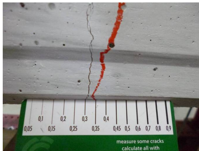
Figure 47. Segment D6: load level of 185 kN, maximum crack width.
