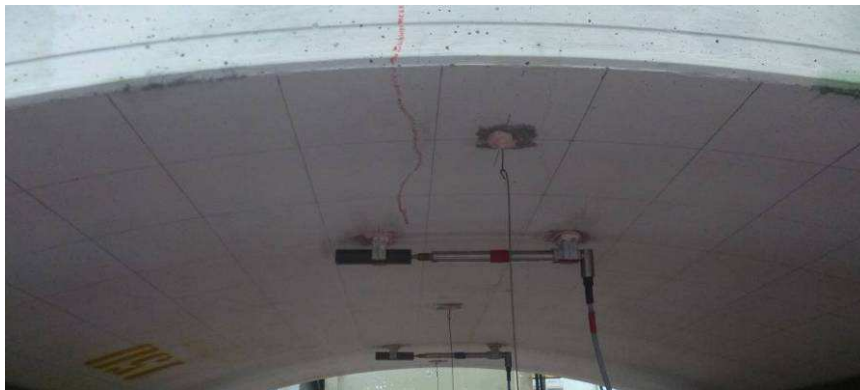
Figure 9. First crack, intrados surface
